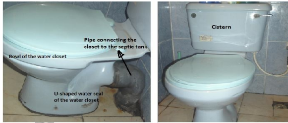
Fig. 2a: Water closet showing the U-shaped water seal and Fig. 2b: Cistern that contains clean water for flushing of pipe connecting the water closet to the septic tank the water closet after use.
